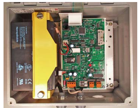
Control Box with Battery
